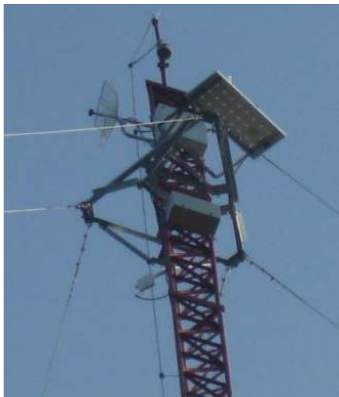
Figure 66. Equipments in a tower.
