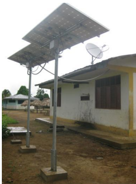
Figure 64. Mechanical support for solar panels.
