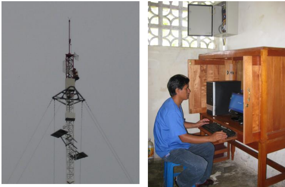
Figure 21. Cabinets on the tower and client station
