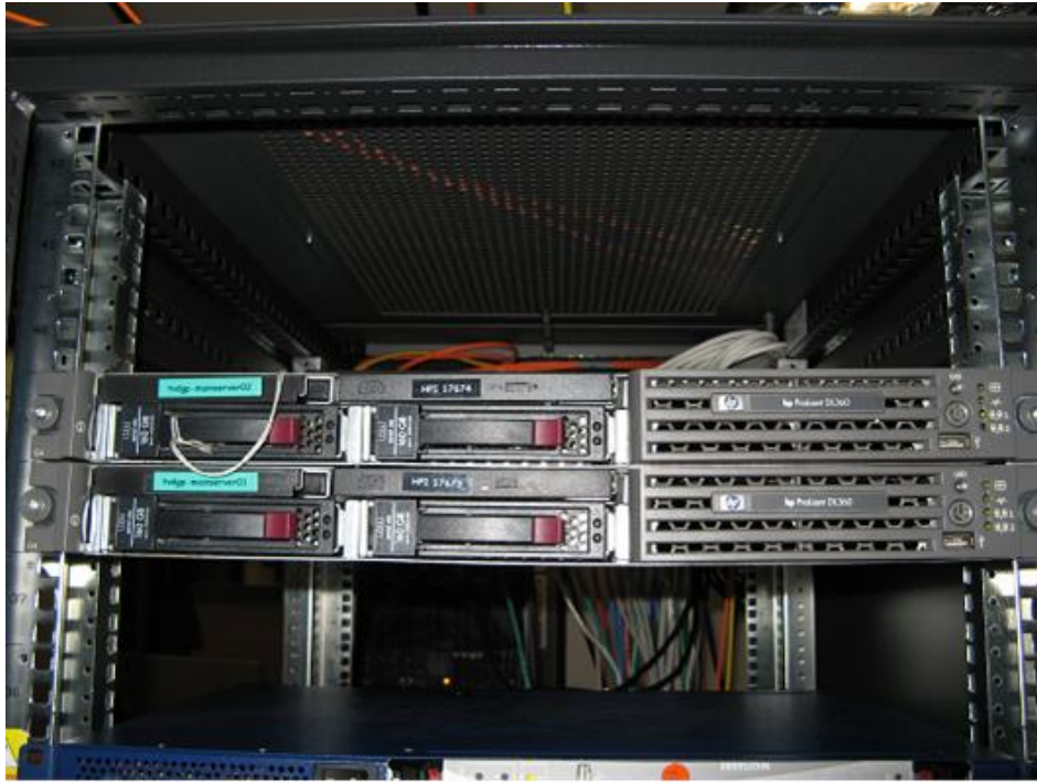
Figure 19: Installed servers for the SVC solution
