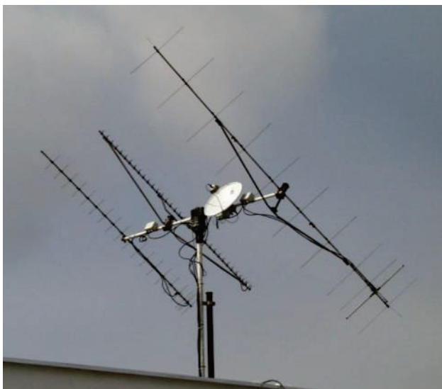
Part of antenna farm
