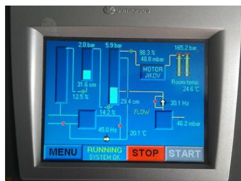
System control interface
