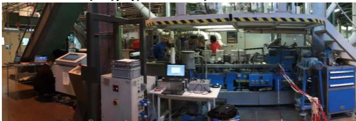
Figure 3.5.3.1 Extrusion line at Addiplast SAS.
