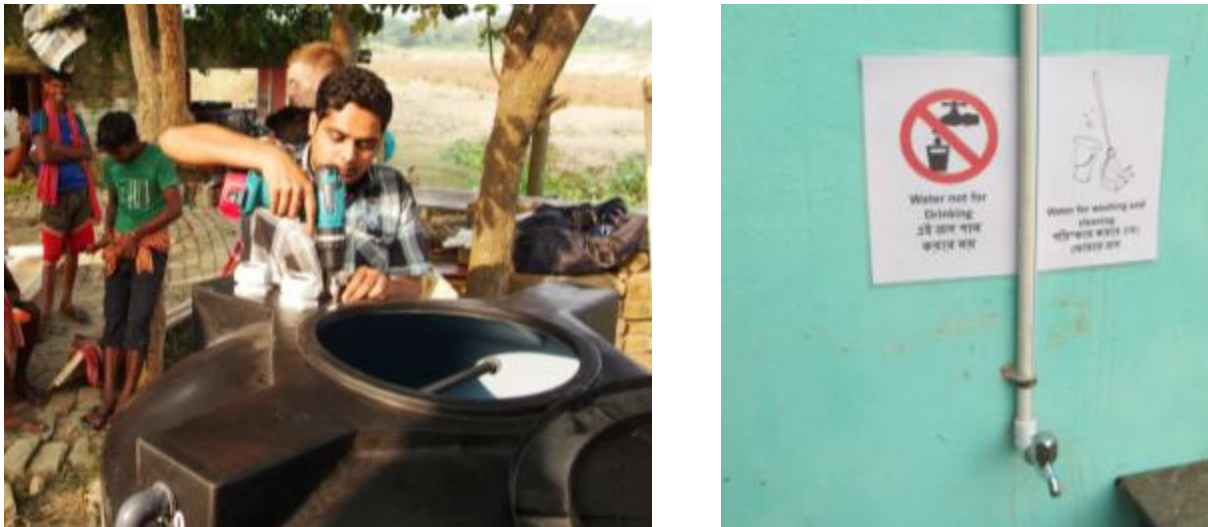
Figure 18: Water tank installation and sampling taps.
