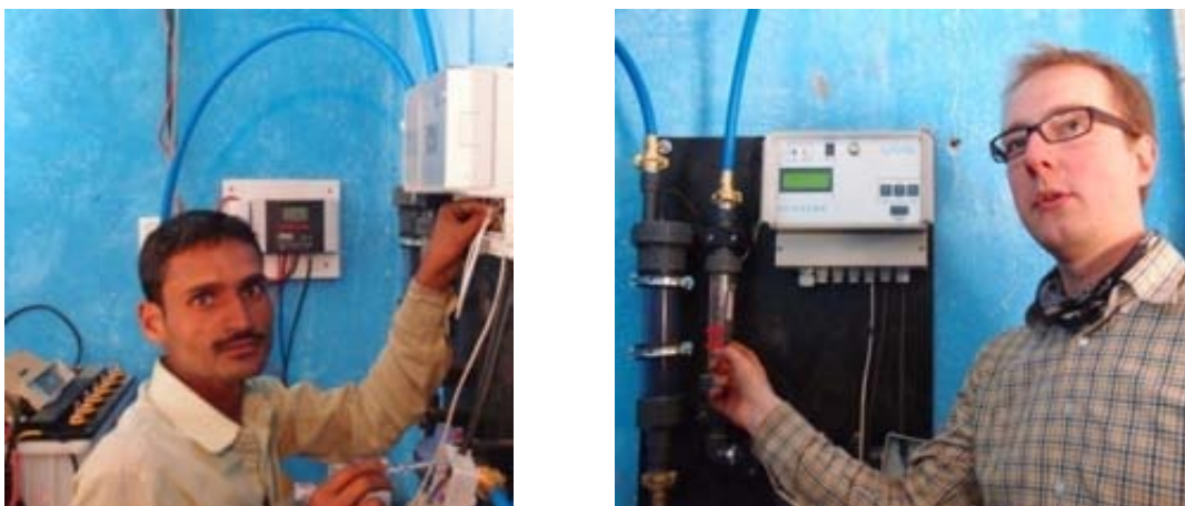
Figure 23: Installation and Explanation of AO Disinfection System.
