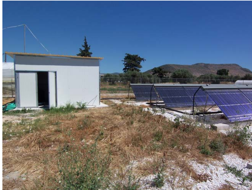
Figure 4. General overview of the installation
