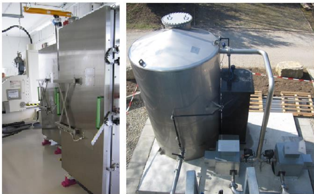
Figure 9 (left) SULFI equipment, (right) waste-gas treatment plant
